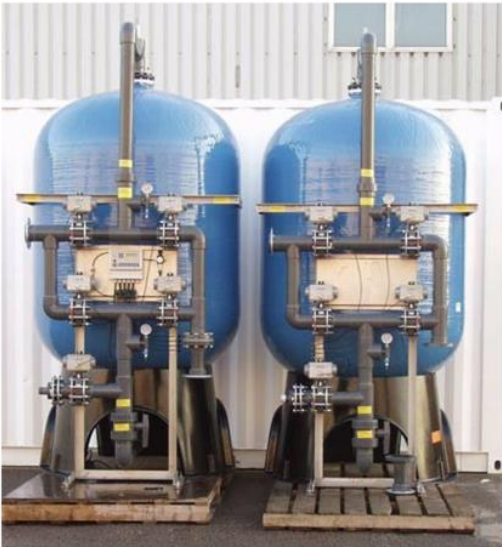
Figure 6: Multi-Media Sand Filtration.
